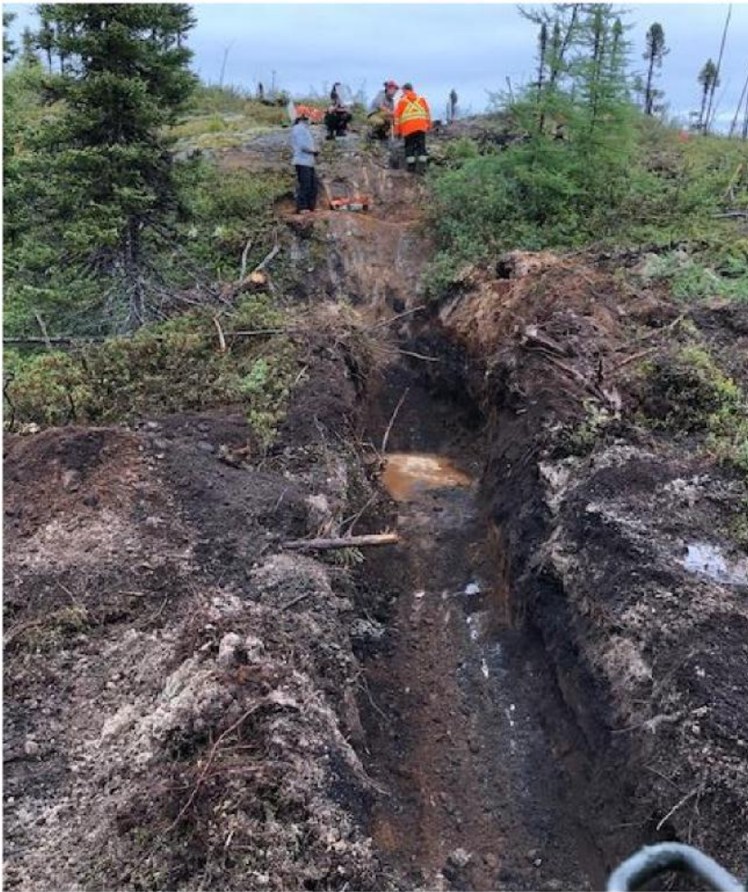
Figure 3: Trenching and sampling being undertaken at the Lac Rainy Graphite Project, Quebec
